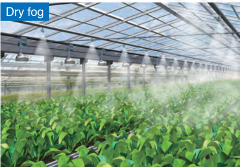
Mist cooling systems
